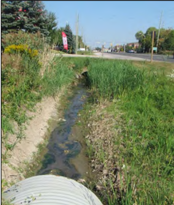
Photograph 41: Drainage in roadside ditch along the north side of Langstaff Road, 200 m west of Dufferin Street, looking east (September 21, 2017).
