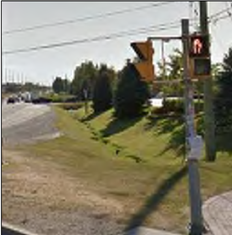
Photograph 45: Roadside ditch on the north side of Langstaff Road west of Dufferin Street, Google Street View from July 2016 shows flow.
