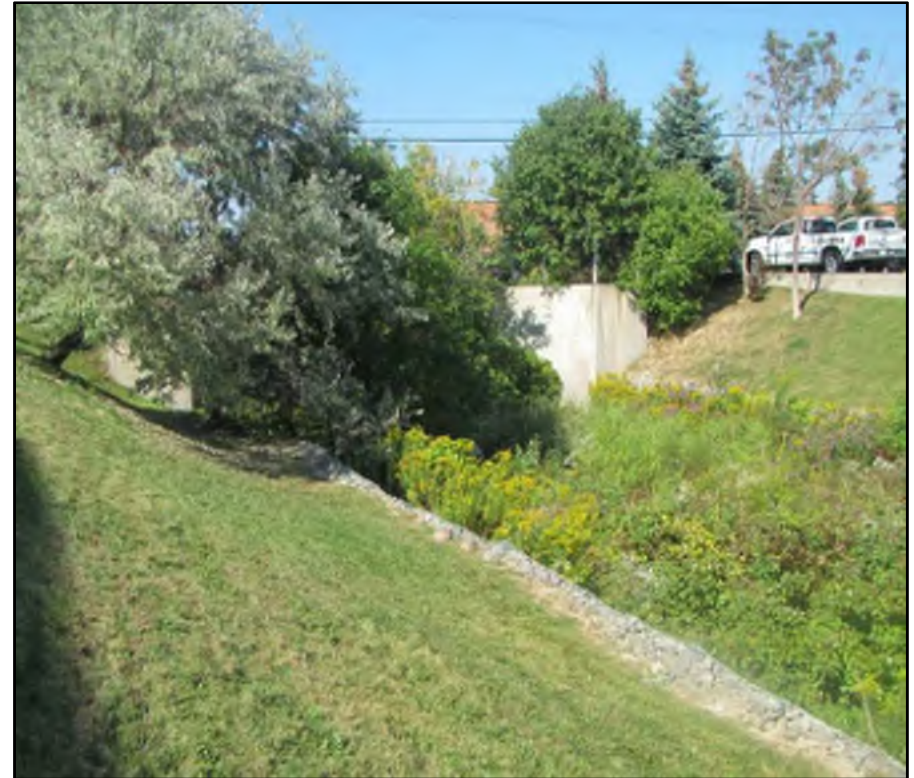
Photograph 40: Westminster Creek culvert, south side of Langstaff Road (September 21, 2017).
