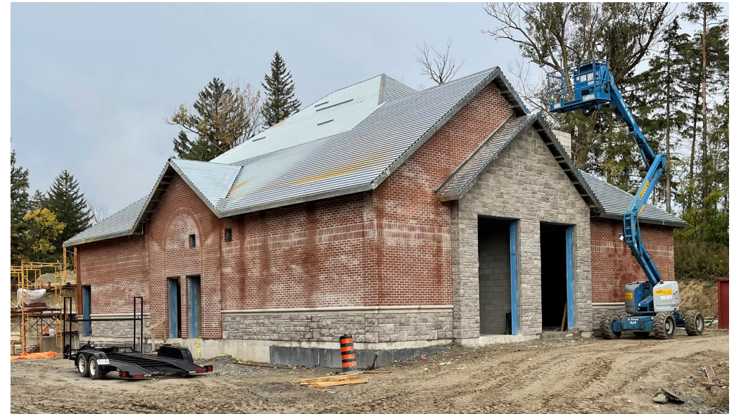
Henderson Pumping Station
