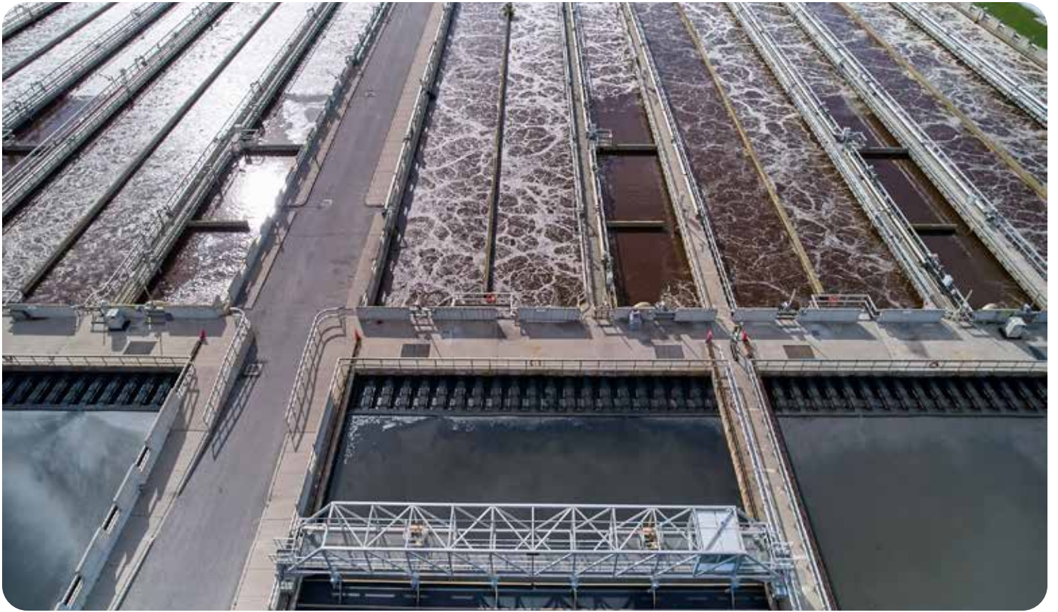
The end of primary clarifier tanks with wastewater continuing to the next process of aeration.
