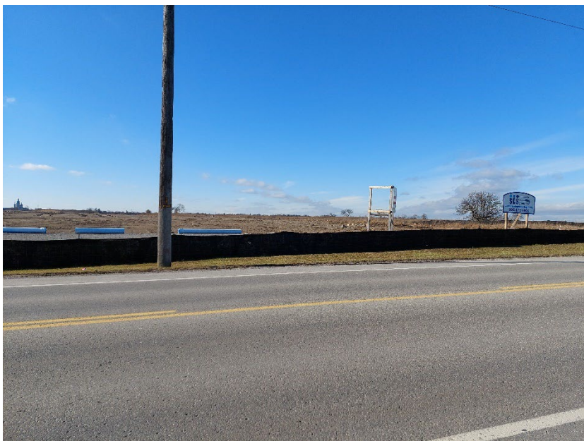
Plate 6: View of construction on the western side of Warden Avenue, looking west-northwest.
