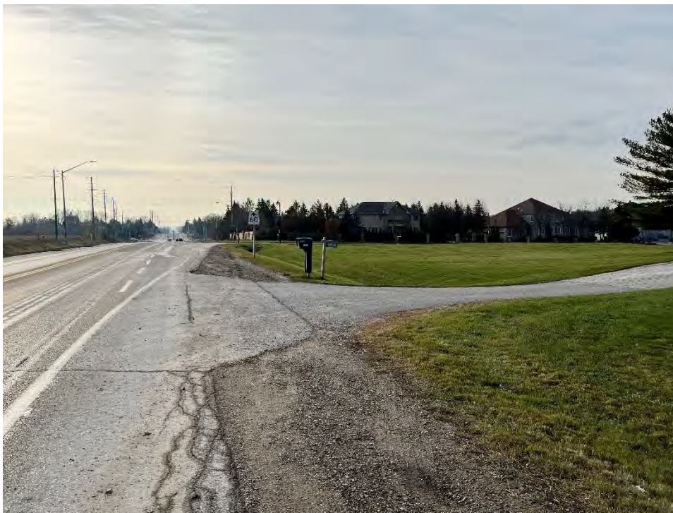
Image 3: Warden Avenue, roadbed and ditch is disturbed. Lands above drainage ditch have potential, require Stage 2 survey.
