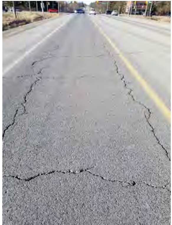
Section 1 – Map cracking
