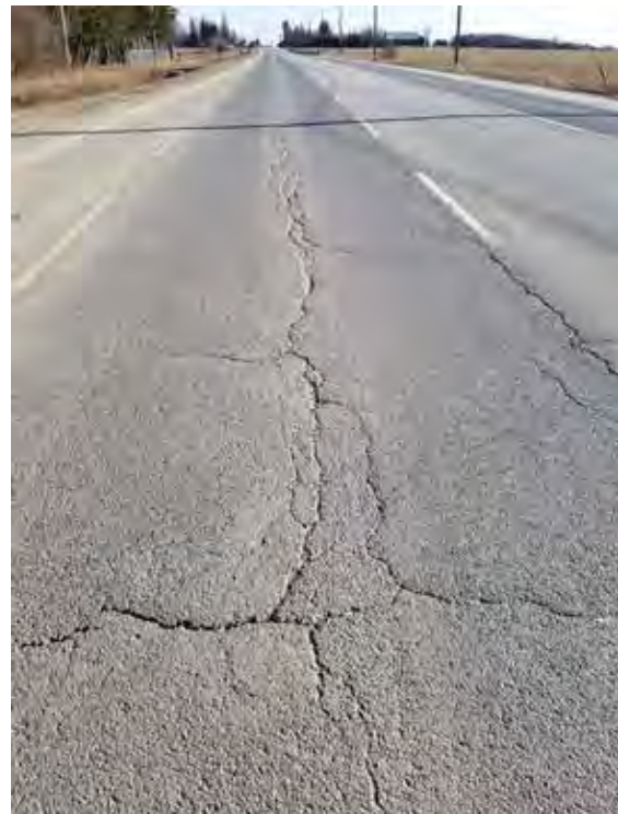
Section 1 – Typical cracking
