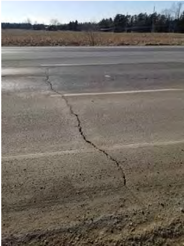
Section 1 – Transverse crack
