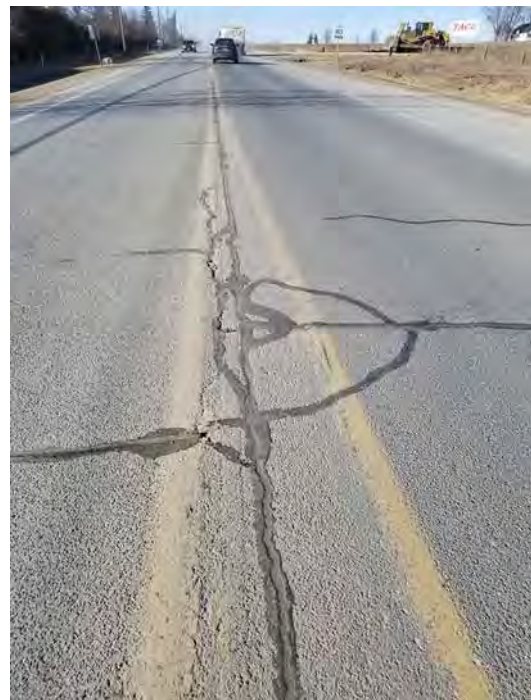
Section 2 – Typical sealed cracks
