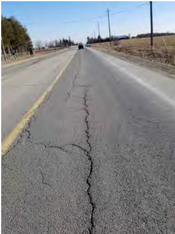
Section 1 – Longitudinal cracking
