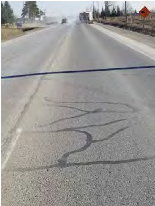
Section 2 – Typical sealed cracks
