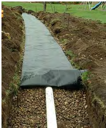
Geotextile being used to prevent fines from entering the trench above. Source: https://wiki.sustainabletechnologies.ca/images/f/5/North_Dakota_State_U_infiltration_trench.jpg
