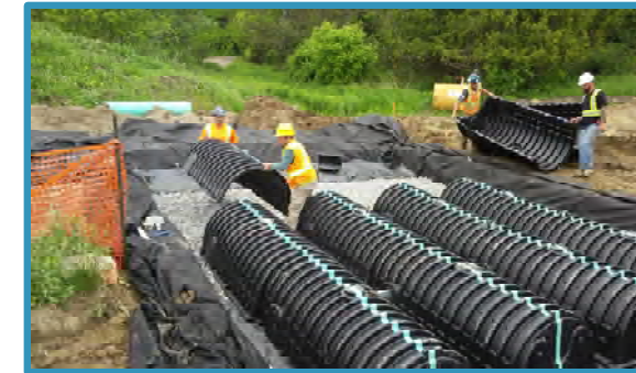
Infiltration chambers being installed. Chamber systems can be large, both in depth and footprint.
