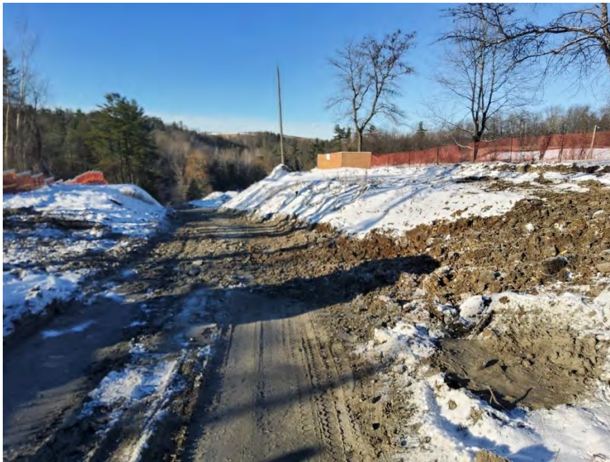
Image 22: Disturbed construction access road and right-of-way associated with the subdivision development at 1600 Teston Road; no potential.
