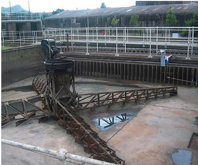
Figure 3-2 Grit Removal Detritor
