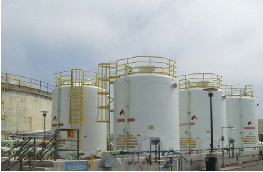
Figure 7-1 Hypochlorite Storage Facility
