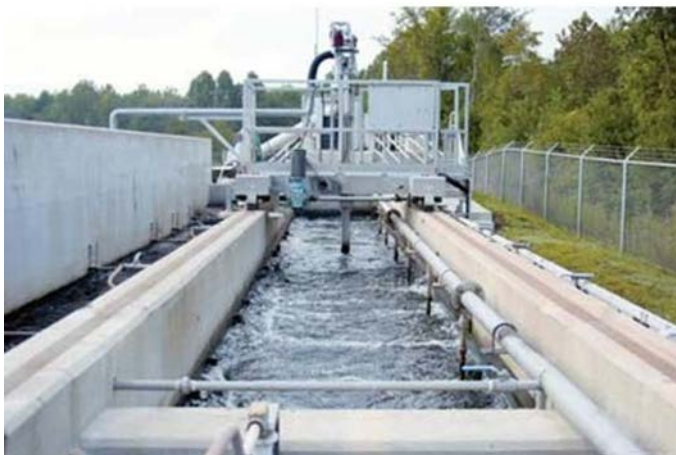
Figure 3-1 Grit Removal Channel
