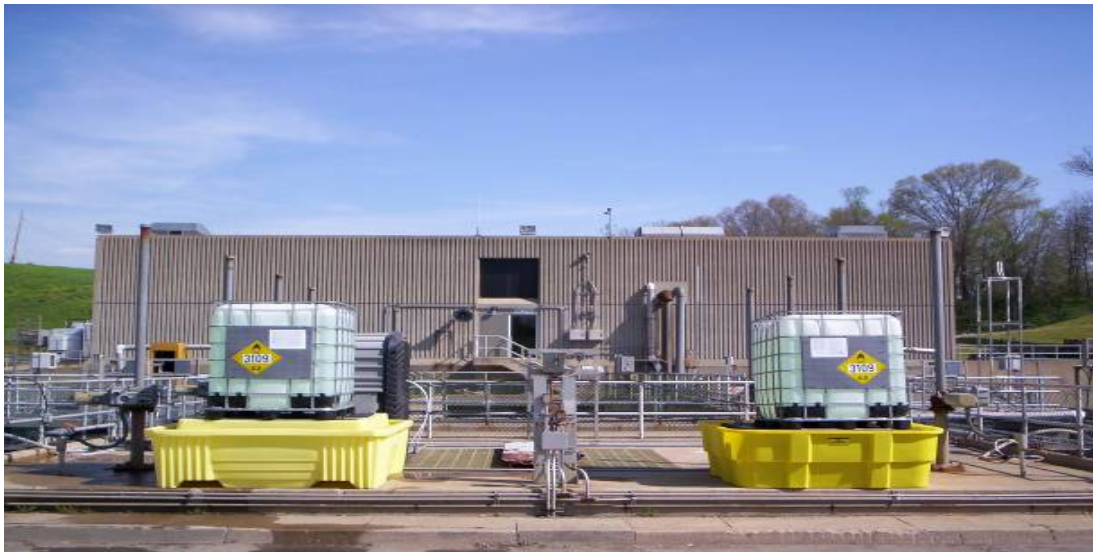
Figure 7-2 PPA Storage Tank Facility
