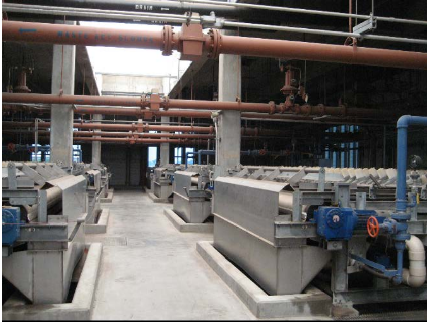
Figure 8-5 Installed Gravity Belt Thickeners at the Bissell WWTP
