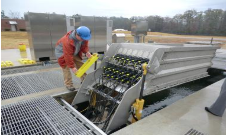
Figure 7-3 UV Disinfection System
