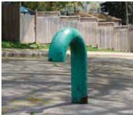
Example of Roadside Watermain Chamber Vent
