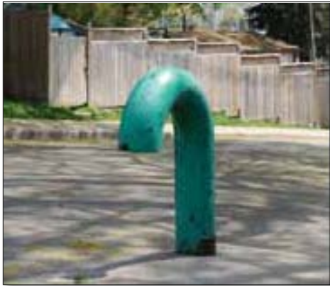
Example of Roadside Watermain Chamber Vent
