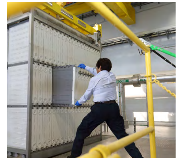
Figure 1 - Water Treatment is an Important Component of the Multi-barrier Approach
