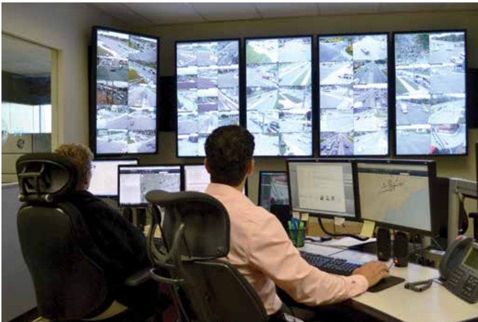
York Region's Centralized Traffic Control Centre
