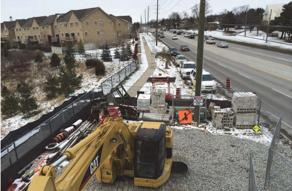
With intensification, working on infrastructure becomes more complex and costly. (Location: North Don)
