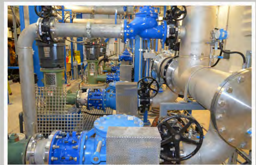
Orchard Heights Pumping Station
