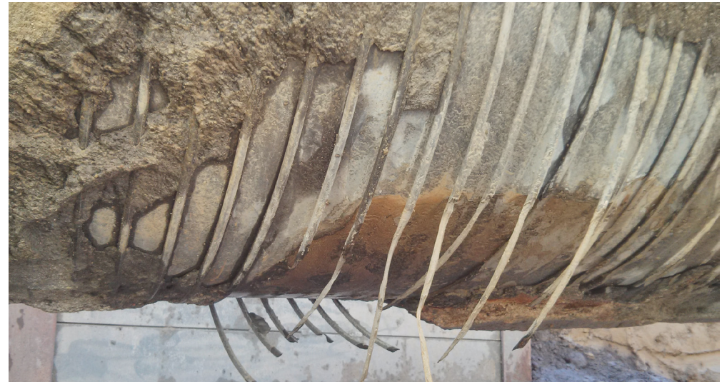
In August 2013, The City of Calgary and Pure Technologies verified distress on a section of BWP on the Memorial Feedermain, finding broken bars and a large area of cylinder corrosion.
