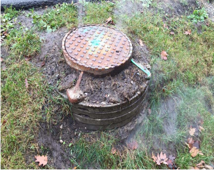
Figure 11 - Smoking Maintenance Hole through Chimney and Frame in Vaughan
