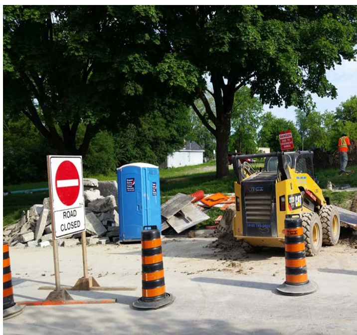
Figure 13 - Lateral Replacement in Aurora
