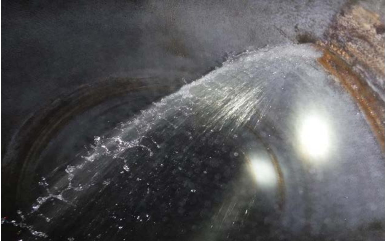
Figure 17 - 16th Avenue Trunk Sewer Gusher Prior to Rehabilitation
